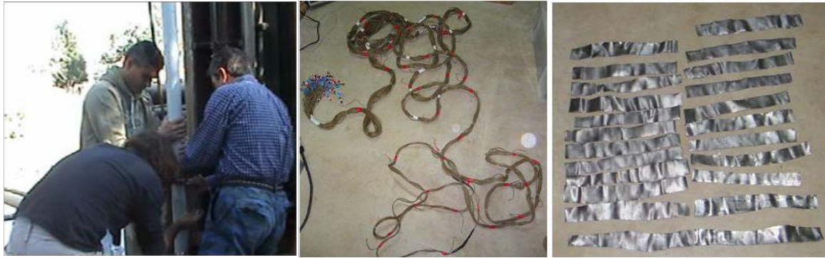
Fig. 2: (left) Installation of the multi-node cable on the outer surface of the plastic piezometer that was placed inside the borehole. (right) Custom made multi-node cable with 48 electrode outputs and lead leaves that were used as borehole electrodes.
