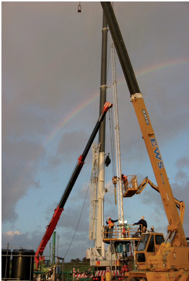
Figure 5. Multi-crane lift deployment of 32 m-long bottomhole assembly consisting of U-tubes, seismic sensors, and pressure temperature sensors at the CO2CRC Otway Project Site, Victoria, Australia.
