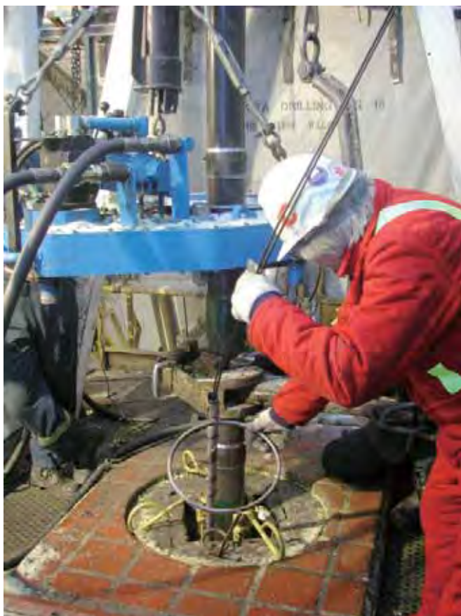
Figure 1. Distributed Temperature Profiling (DTS) fiber-optic cable installation for permanent temperature surveys behind the casing at Mallik Gas Hydrate drilling site in Canada. Fiber-optic cables are attached to the outside of the casing wall by special cable clamps to prevent cable damage while running into the hole. Special cable outlet connectors at the well head ensure safe data retrieval from the cemented borehole annulus to the surface.
