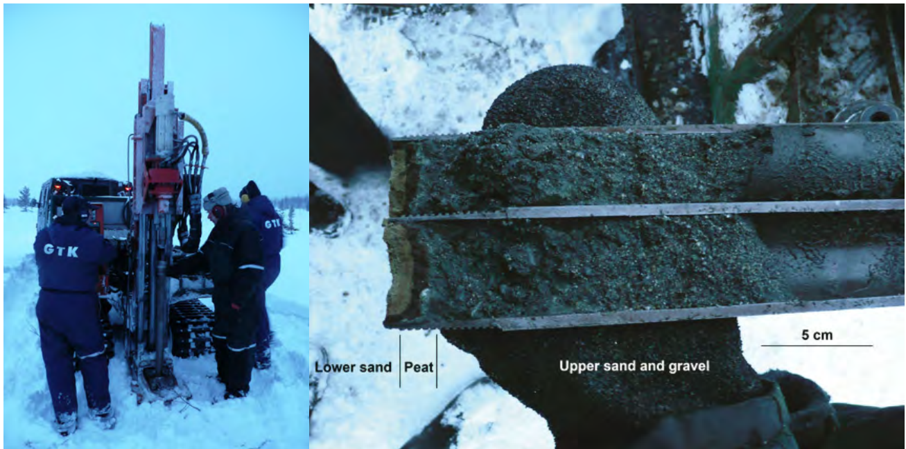
Fig. 2. a) Percussion drilling in Järämäapa and b) longitudinal section of 3.5 cm diameter percussion drilling core from Järämäapa, showing the 1 cm thick organic layer between sands and gravels (January 2008. Photos: P. Sarala).
