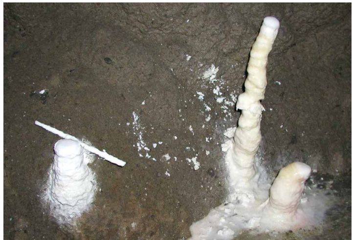
Figure 6.9.6. Calcite stalagmites growing on the floor in blasted and concreted section of the Bedřichov water-supply tunnel section A. Photo J. Klomínský. (Size of the largest stalagmite is about 30 cm.)
