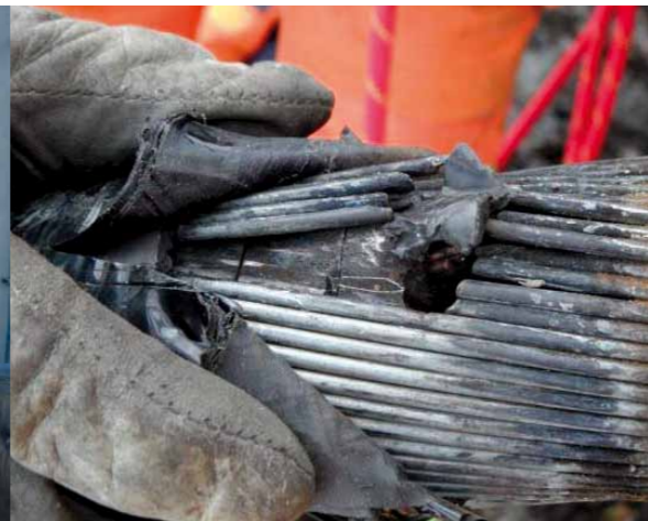
Schadhafte 20-Kilovolt-Leitung 20 kilovolt mains supply had broken down
