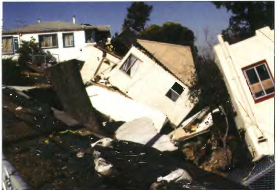
Structures destroyed by a landslide along 19th Street in Oakland, Calif. The landslide extends from the left side of the photo, downslope to the right. (Photo: USGS/J. Coe)
