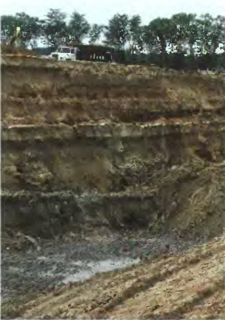
Figure 4. Commercial solid-waste disposal facility in the Patuxent River valley. Understanding the geology of Coastal Plain deposits in this area helped locate clay beds forming the impermeable boundary at the bottom of the pit. Photo by W.L. Newell.
