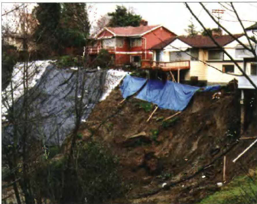
Landslide in northwest Seattle. The foundation of the house at far right and decks of neighboring houses were undermined. (Photo: Al Chleborad, USGS)
