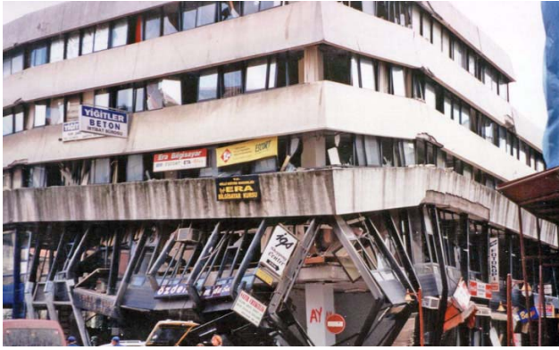
Fig. 1. A seriously damaged RC building in Marmara region.
