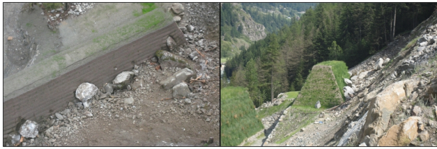
Fig. 1. Example of rock elements stopped by a reinforced embankment (Aosta Valley, Italy) (courtesy Officine Maccaferri S.p.A.).
