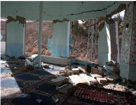
Fig. 6. Various damages after the earthquake (Naseer et al., 2007; Khan and Khan, 2008).
