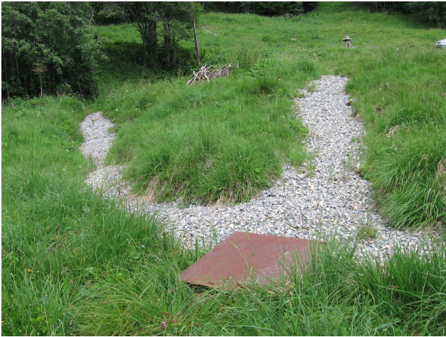
Fig. 19. Enclosing structures: Drainage system to stabilise the sliding layers of the slope.
