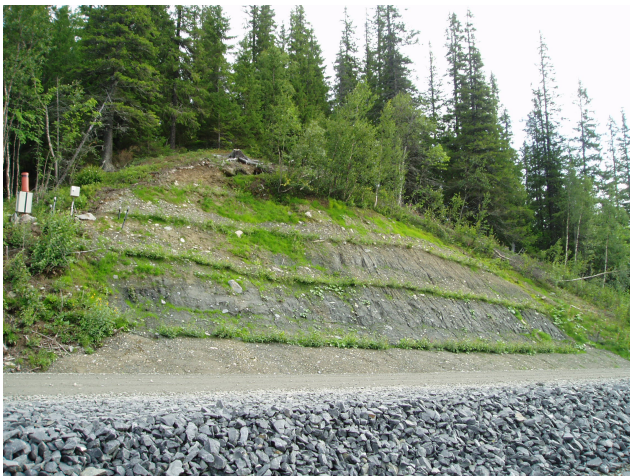
Fig. 17. New building and upgrade: Soil bio-engineering measures to stabilise unsteady slopes (courtesy of: Rankka, 2005).
