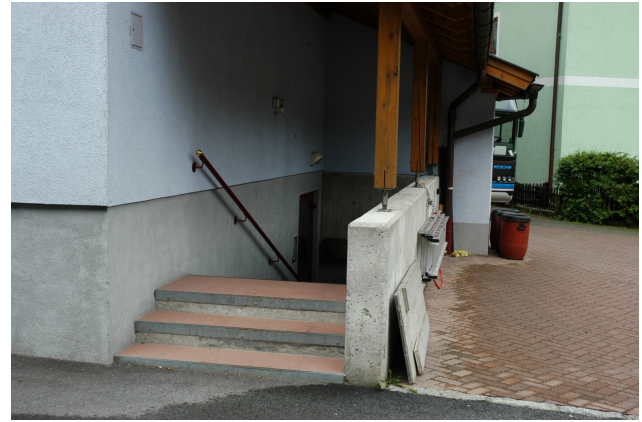
Fig. 10. New building and upgrade: Enhancement (raising) of base-ment stairs above flood level.
