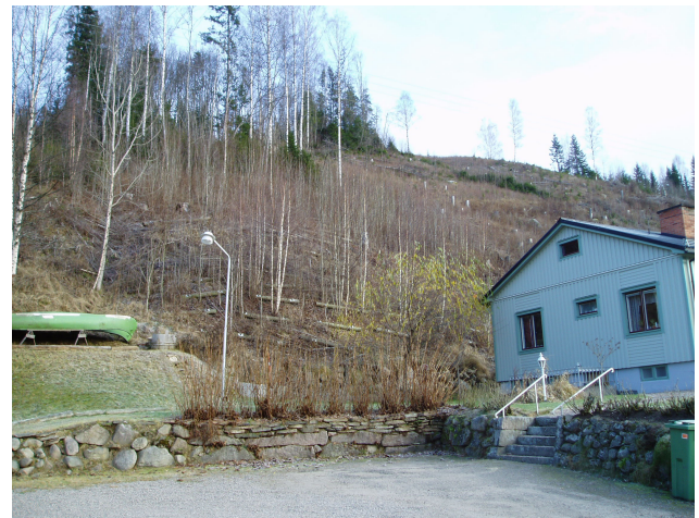
Fig. 18. New building and upgrade: Soil nailing measures to stabilise unsteady slopes (courtesy of: Rankka, 2005).
