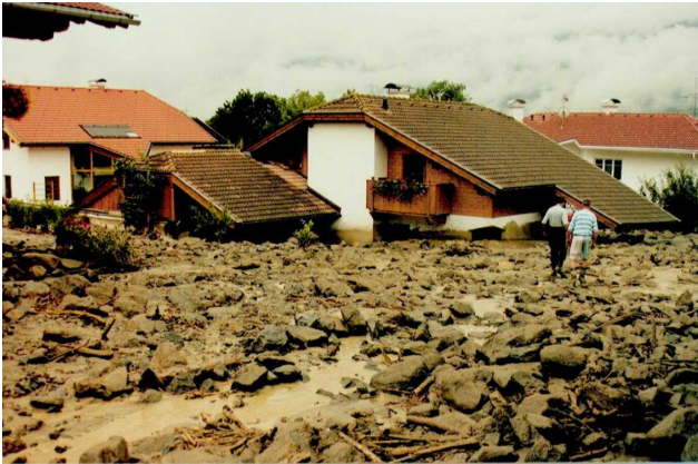
Fig. 2. The debris flow event of 16 August 1997 damaged buildings situated on the Wartschenbach fan, community of Nußdorf-Debant, Austria.
