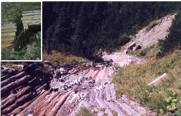
Fig. 2. The wooden drainage system is disrupted by the eroding power of debris flows, by small slides from the adjacent slopes (top right) and by differential movements within the landslide (detail top left), which leads to increased displacements rates.
