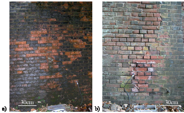
Fig. 1. Weathered walls of one of the tunnels of Usui Pass railway. (a) Bricks of north-facing walls are fractured by frost action. (b) Bricks of south-facing walls are weathered by salt efflorescence.
