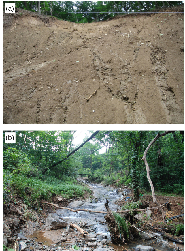
Figure 5. Landslides in Site B. (a) A closer look of the landslide initiation zone. A small volume of soil slid down along the smooth clayey surface which acts as a slickensided shear plane. (b) Upstream valley where debris flows were traced, looking northwest.
