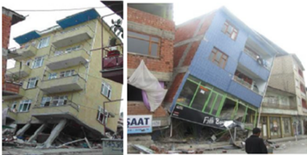
Figure 8. Examples of damage related to soft-story and weak-story irregularities (source: Ahmet Topçu).
