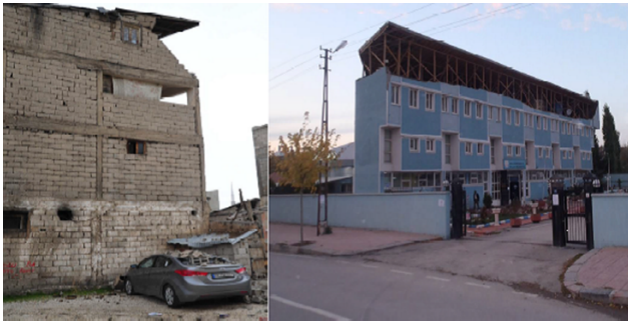
Figure 23. Gable wall damage (www.dramaistanbul.com.tr).
