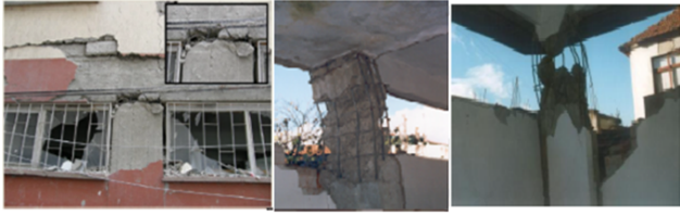
Figure 6. Examples of damage caused by the formation of short columns (METU/EERC, 2011).
