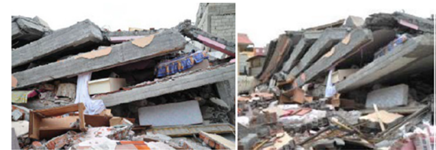
Figure 19. Full collapse of a building as a result of plastic hinges in the bottom and top zones of columns in a reinforced concrete structure in Van-Ercis (Onen et al., 2011).
