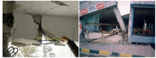
Figure 11. Pulling away of longitudinal reinforcements.
