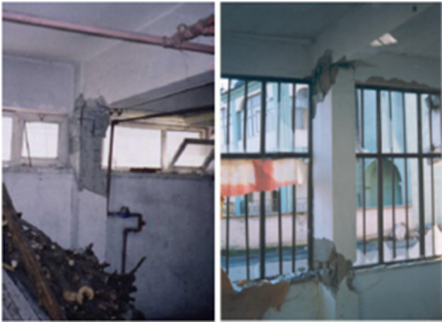
Figure 7. Short column formation caused by ribbon windows (METU/EERC, 2011).
