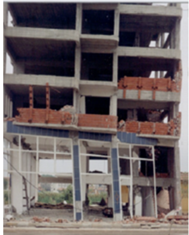
Figure 9. Heavy damage in the weak story of a five-floor building in Adapazari (17 August 1999 Kocaeli earthquake, M = 7.4 ) (Isik G., 2006).
