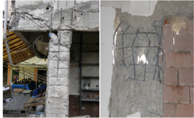
Figure 14. Damage caused by excess stirrup intervals in the confinement zones of columns (Onen et al., 2011).
