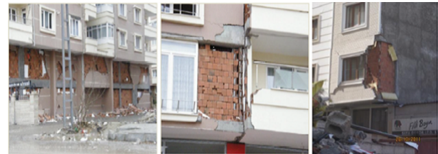
Figure 26. Damage in the outer walls of a reinforced concrete building in Van city due to separations in the walls (Cagatay I.H., 2007).
