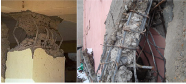
Figure 13. Damage caused by reinforcement detailing mistakes (Source: Erdal Camci).
