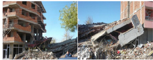
Figure 25. Reinforced concrete multi-story building that collapsed by colliding with adjacent buildings due to a hammering effect (Inel et al., 2011).
