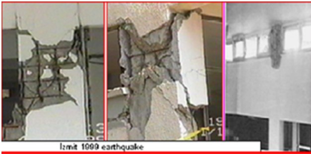
Figure 3. Several short column failures observed after earthquakes (Isik G., 2006).
