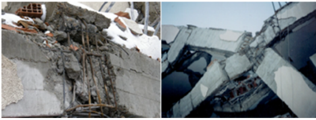
Figure 16. Damage to column-beam joint region (Onen et al., 2011).
