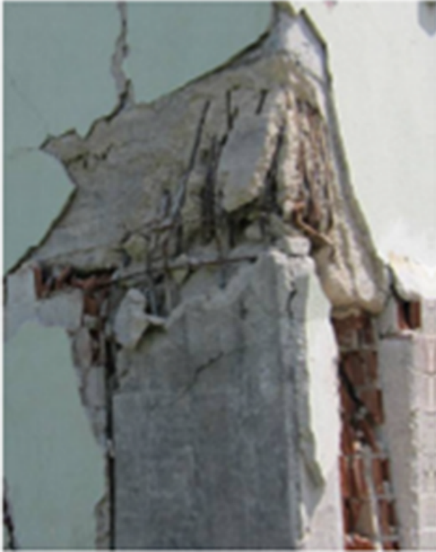
Figure 10. A reinforced concrete structure that was heavily damaged at the joint region during the 19 May 2011 Simav earthquake (Cayci, 2012).
