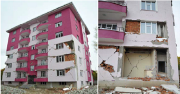
Figure 22. Damage observed in non-bearing brick-infilled walls.
