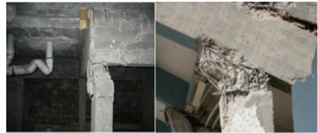
Figure 18. Examples of strong-beam-weak-column damage.
