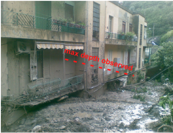
Figure 6. Evidence on the wall of the maximum depth observed during the event.
