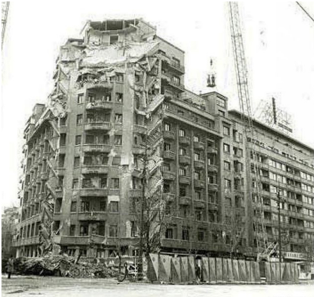
Figure 7. Wilson block of flats after earthquake (1977). Source: courtesy of Rezistența urbană (Urban resistance).
