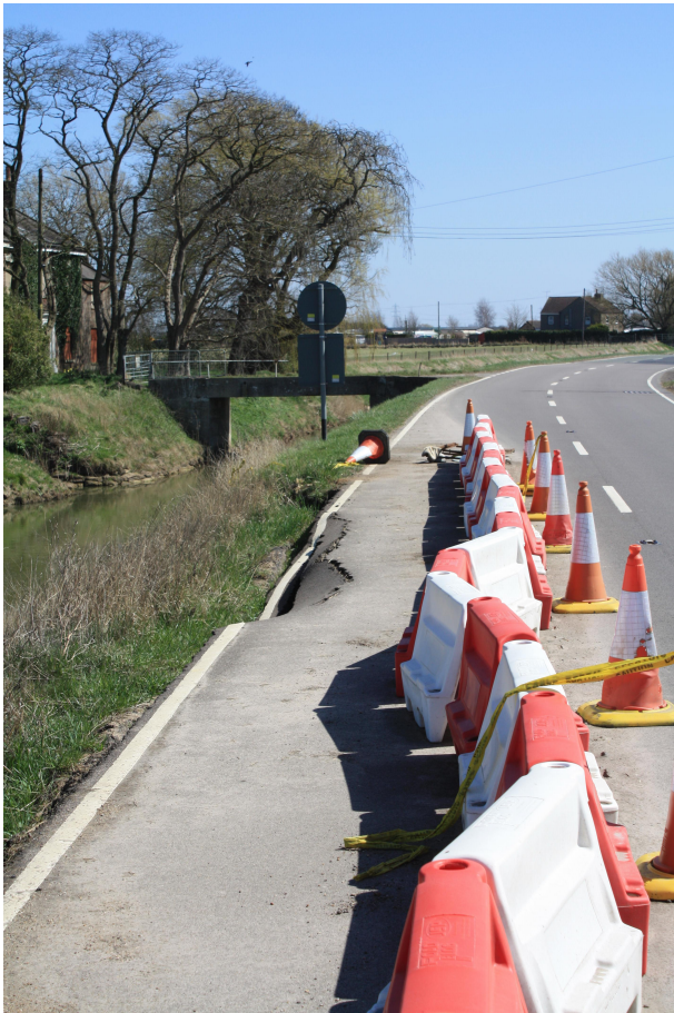
Figure 8. Road embankment instability, B1165 Ravens Bank, Lincolnshire (photo: O. Pritchard).
