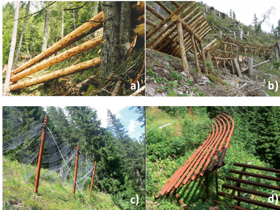
Fig. 2. Avalanche protection measures: (a) wooden stems, (b) wooden grills, (c) steel nets, and (d) steel bridges. (Photos (a) and (b): Forestry Department of Canton Berne, Natural Hazards Division, Interlaken.)
