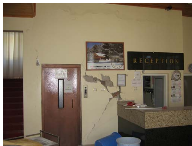
Fig. 10. Filled wall damage.
