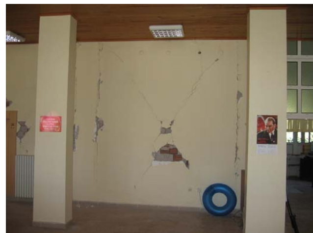
Fig. 9. Filled wall damage.
