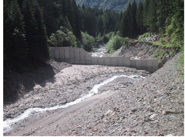
Fig. 7. Fresh debris-flow deposits above the partially built check dam near the sensor S1 (see Fig. 2 for location).
