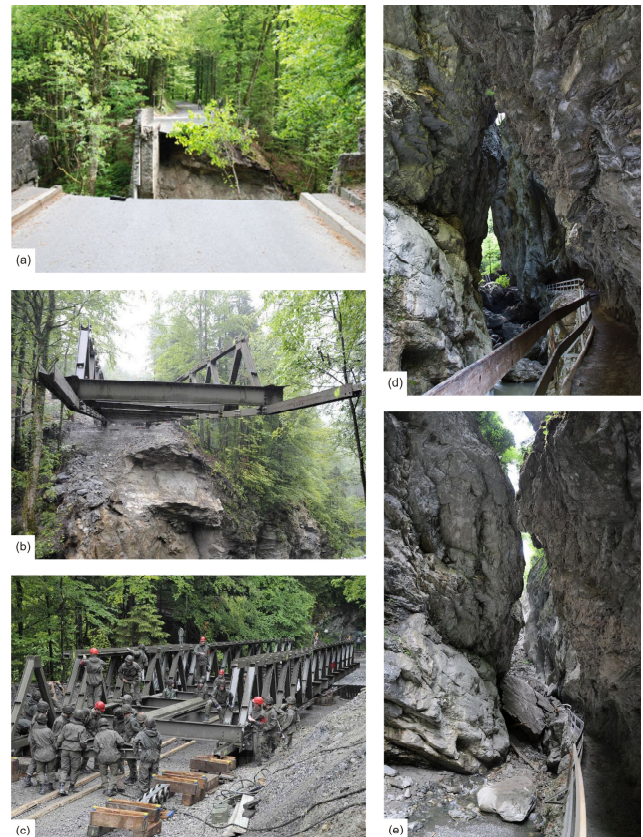
Fig. 2. Impact of the destructive rockfall: (a) the destroyed bridge (photo: Stefan Hoch, source: www.bmlv.gv.at ); (b and c) reconstruction of the bridge by the Federal Armed Forces of Austria (photos: Sigi Schwärzler, source: www.bmlv.gv.at ); (d) view into the gorge in 2010 before the rockfall occurred (photo: Bernhard Mäser) and (e) two days after the rockfall event on 12 May 2011 (photo: Friedrich Böhringer).
