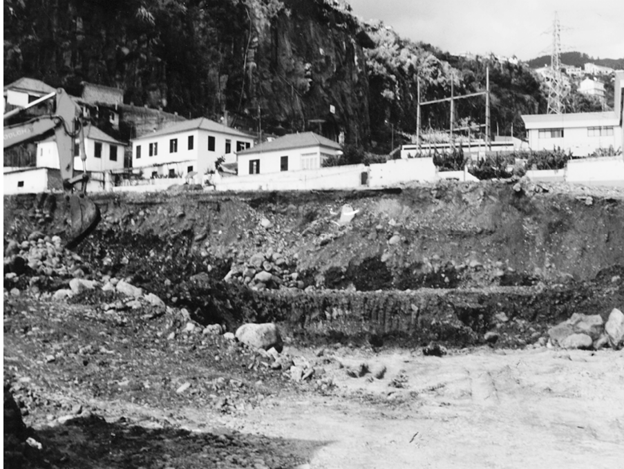
Fig. 8. City of Funchal: excavation works to make a new building area removing the support of the area already built (image taken by the author).
