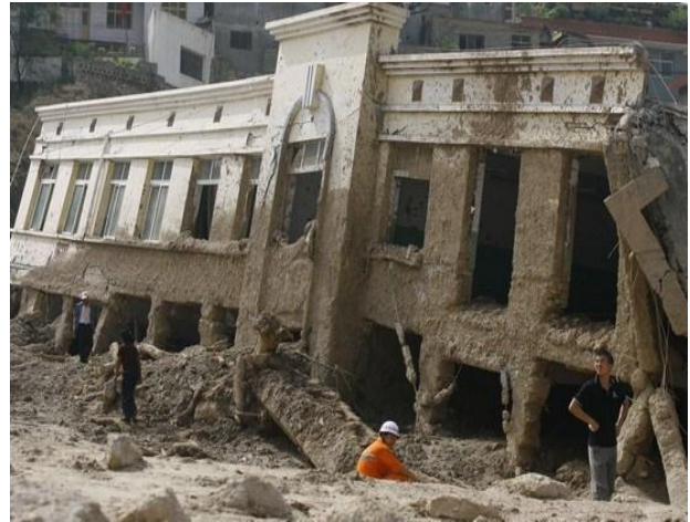
Fig. 14. A two-storey building was totally destroyed due to the direct impact of debris flow. Mud trace still remained on the wall of the building.
