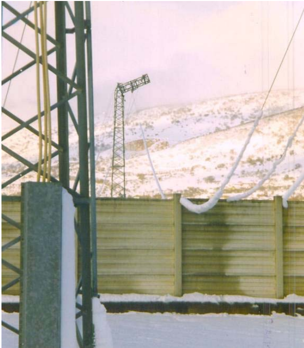
Fig. 2. Tower collapse due to overload ice on conductors during a wet snow event (Puglia – Italy; winter 1995).
