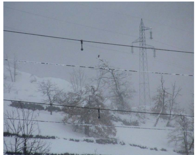
Fig. 1. Counterweights on a 132 kV power line limit the wet snow accretion on wires (Valle Stura – Piedmont – Italy; 19 February 2010).
