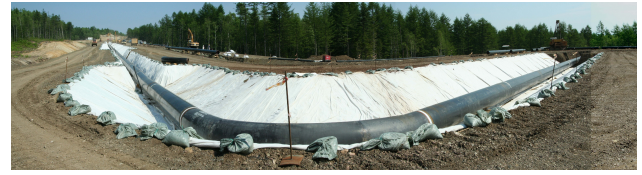
Fig. 2. Construction of the dog-leg structure at the trunk pipeline/active fault crossing at Sakhalin. Photo courtesy Oksana Golubtsova.
