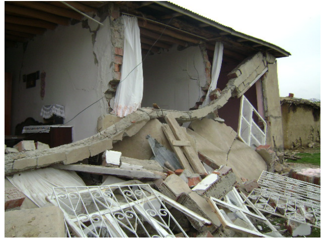
Fig. 10. Out-of-plane failure due to long span.
