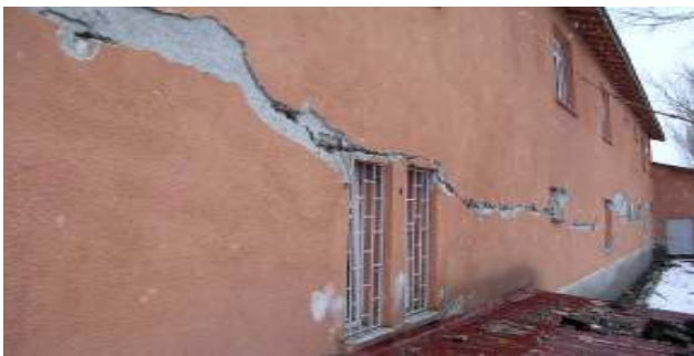
Fig. 6. Cracking of masonry wall with many openings (Erzurum, 2004) (Source: A. Turer).
