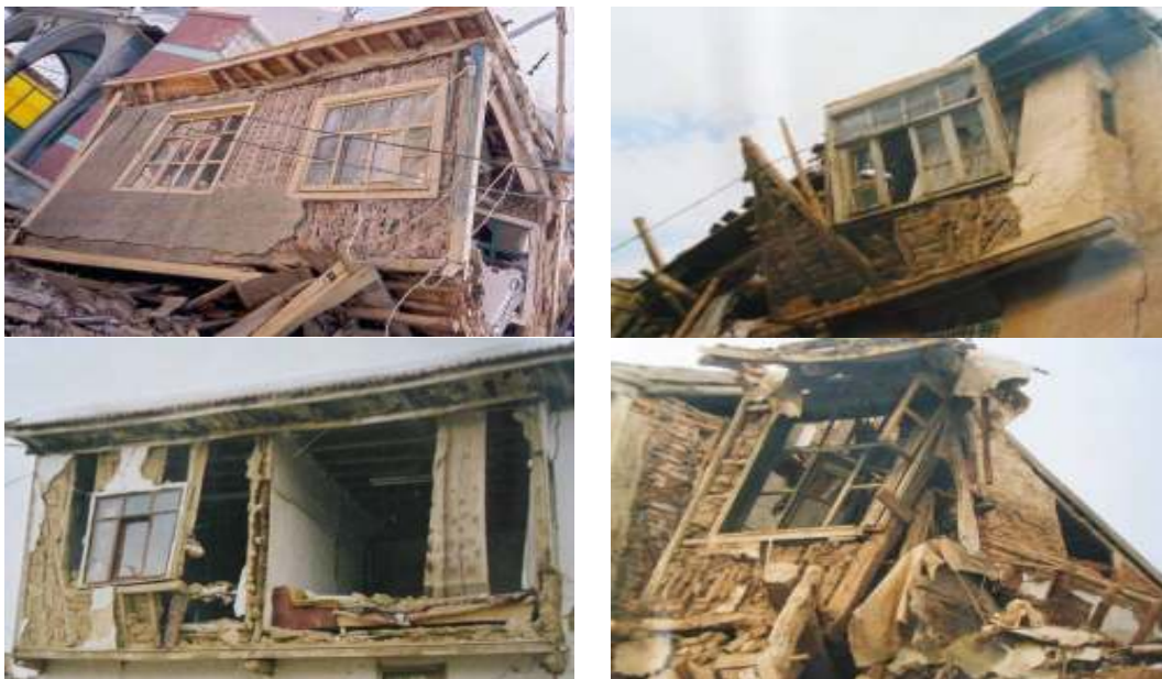
Fig. 25. Failure and damage of himis buildings (Source: D. Aydin).
