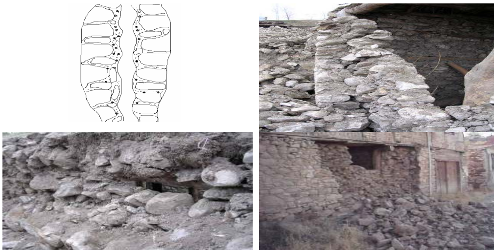
Fig. 19. Wall delaminated with buckled skins (Source: T. Wasti).
