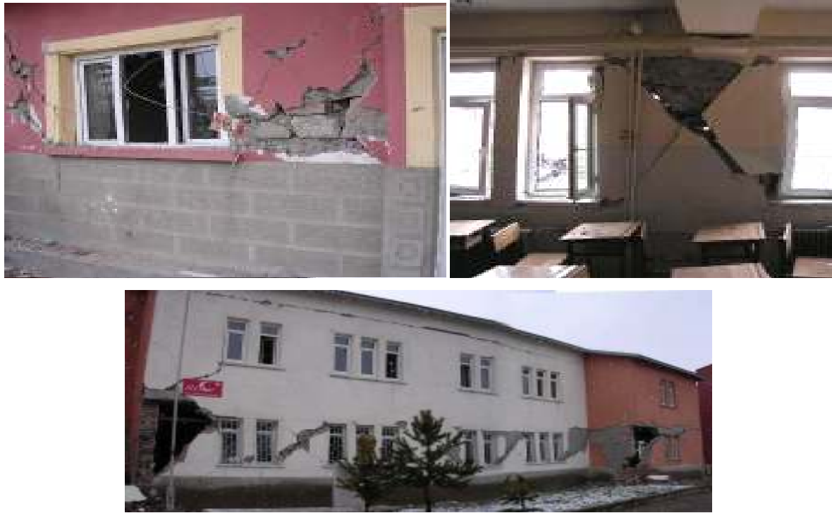
Fig. 10. Shear cracks of piers between windows (Erzurum, 2004) (Source: A. Turer).
