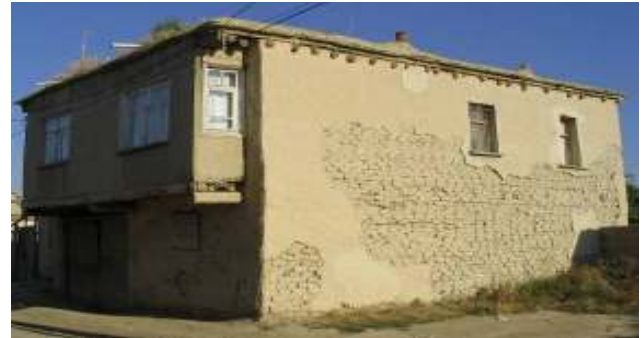
Fig. 23. A kerpik structure in Aksehir with two storeys and absence of hatil (Source: H. H. Korkmaz, S. Z. Korkmaz, M. S. Donduren).
