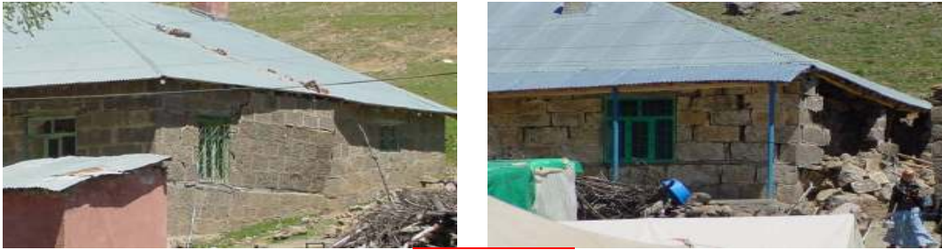
Fig. 20. Failure of block stone masonry houses (Source: A. Turer).
