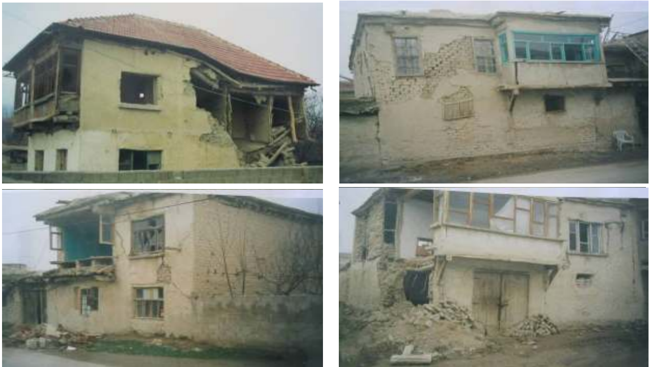
Fig. 11. Damage of multistory houses (Source: D. Aydin).
