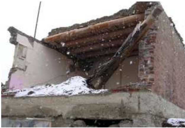
(a) Out-of-plane collapse of the walls (Source: A. Turer)
