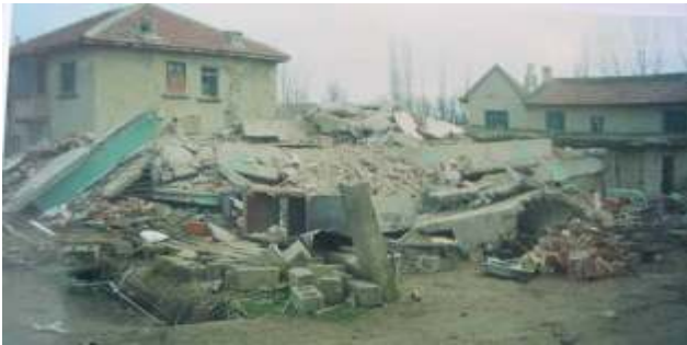
Fig. 22. Collapsed reinforced concrete building after Sultandagi earthquake (Source: H. H. Korkmaz, S. Z. Korkmaz, M. S. Donduren).
