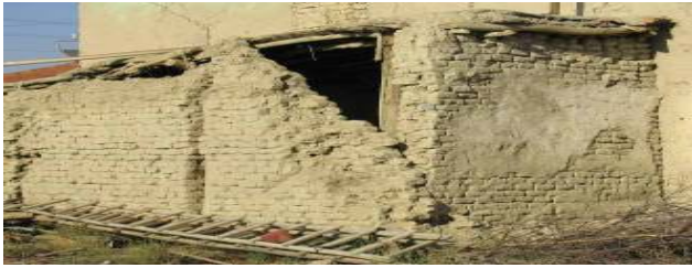
Fig. 9. Inadequate (no) connection between two intersecting walls and damage (Source: H. H. Korkmaz).
