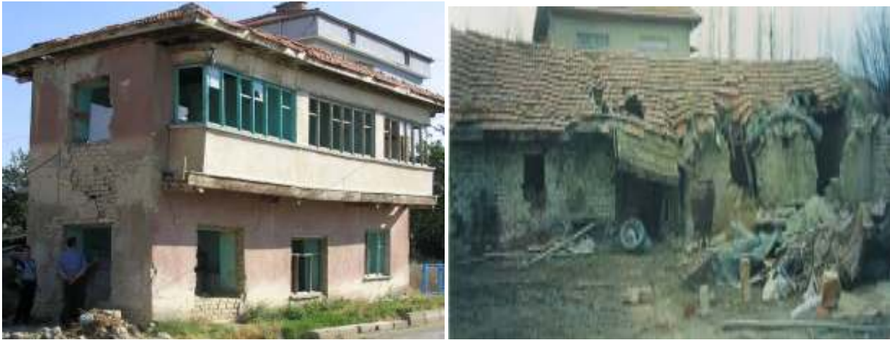
Fig. 12. Failure of structures with bad geometry (Aksehir, 2003) (Source: H. H. Korkmaz, S. Z. Korkmaz, M. S. Donduren).
