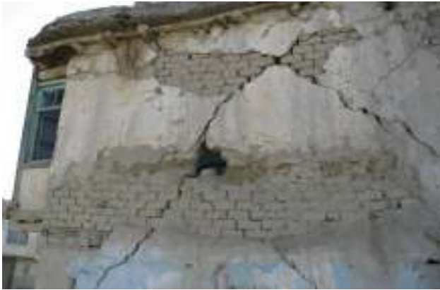
(c) Diagonal shear cracking (Source: H. H. Korkmaz)
