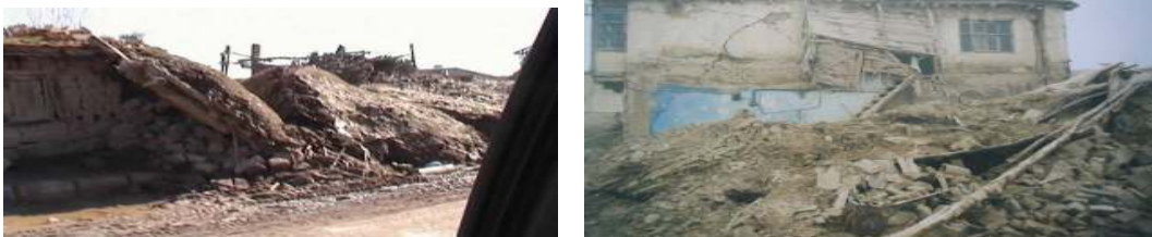
Fig. 21. Failure of heavy roof of kerpik houses (Sultandagi Earthquake) (Source: D. Aydin).
