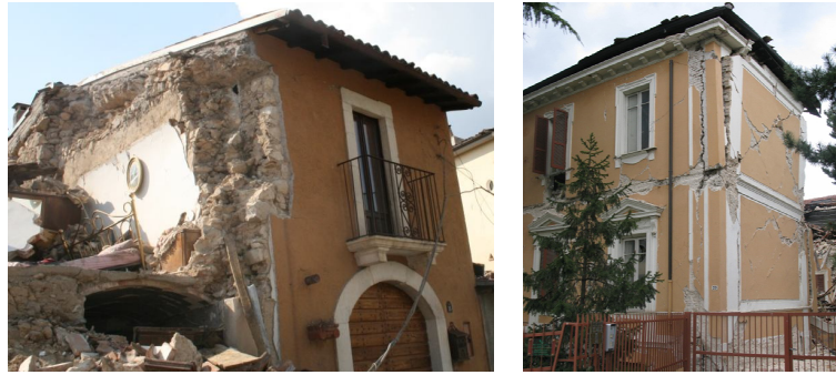
Fig. 12. Badly connected crossing walls causing out-of-plane failures.
