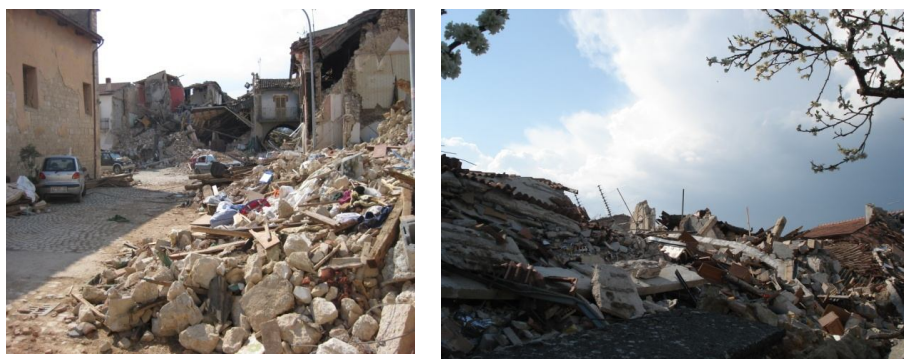
Fig. 2. A general view of building damage in Onna; collapsed and severely damaged residential buildings.
