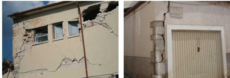
Fig. 13. Damages observed at connection of crossing walls.
