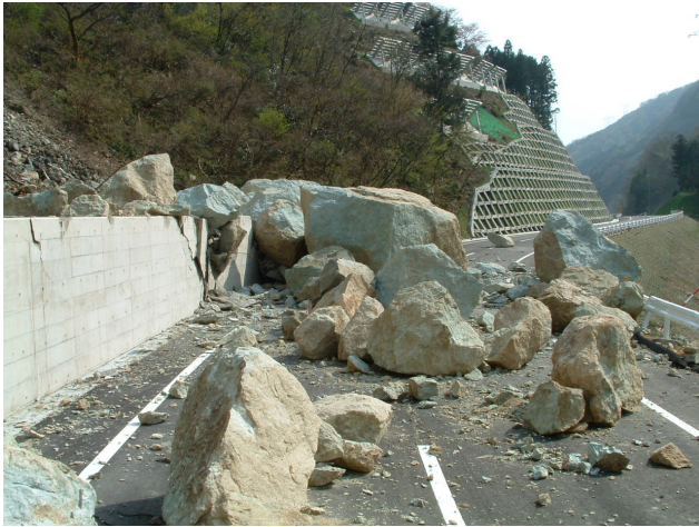
Fig. 1. Rockfall event on road N364, Kaga, December 2004.
