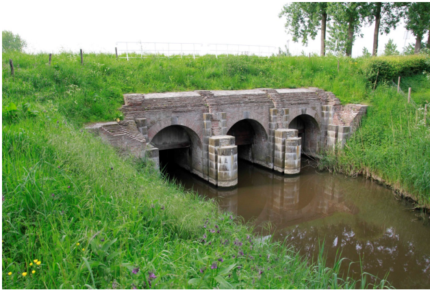
Figure 5. Land side of an inundation sluice, built in 1789 by the Estates General of the Dutch Republic at Zwartenhoek (51°15' N and 3°51' E). Notice the double groove in the protruding parts in which beams could be installed. As the space in between the beams could be filled with earth, this construction was strong enough to prevent the fresh water from flowing seaward. After some weeks water in polders could reach a level of some decimetres. As soon as the threat of war disappeared, beams and earth were removed again (photo: Nellie de Kraker).
