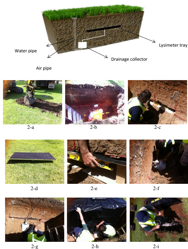
Fig. 2. Pan lysimeter installation, (a) trench excavation, (b) cavity digging, (c) cavity levelling, (d) lysimeter tray, (e) placing the tray, (f) placing the collecting bucket and connect the tray and bucket by a PVC pipe, (g) PVC pipe and access tubes, (h) plastic sheet for protecting the cavity, (i) compacting the backfilled soil.
