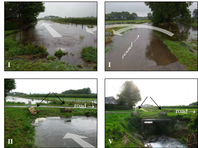
Fig. 12. The role of culverts during the 27 August 2010 flash flood. The roman numerals indicate the post-event field surveys (Table 1). Upper panels: Situation directly after the flood. Upwelling water reveals the exit of the submerged culvert. The resulting backwater feedback allows water to bypass the obstacle on the right by flowing over the road and the adjacent field back into the brook (arrows). Lower left panel: upstream entry of the culvert. Logs (black arrows) deposited by flood and flow marks in grass (upper left panel) indicate that water flowed over the culvert at flood peak. Lower right panel: situation two weeks after flood with flood marks indicated. The photos in the top panels of Fig. 8 are taken from the same location as the photos in this figure, but in upstream rather than downstream direction.
