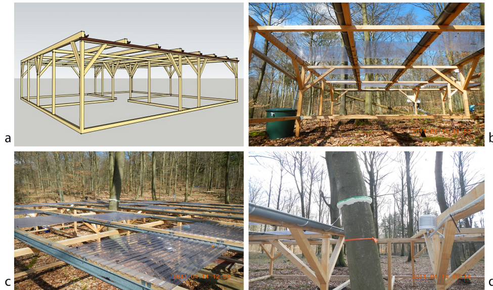
Figure 3. Roof construction sketch of the main roof (10 × 10 m) (a). Roof with panels, rain gutters, water barrel and main tree (b, c). Roof detail with main tree and stem rim to collect stem flow (d). All pictures were taken at plot SEW48.
