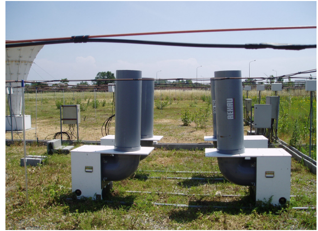
Fig. 2b. Same as Fig. 2a by replacing the iron elbow by a PVC one and 1-m extension allowing 6 dB attenuation at the ground level.
