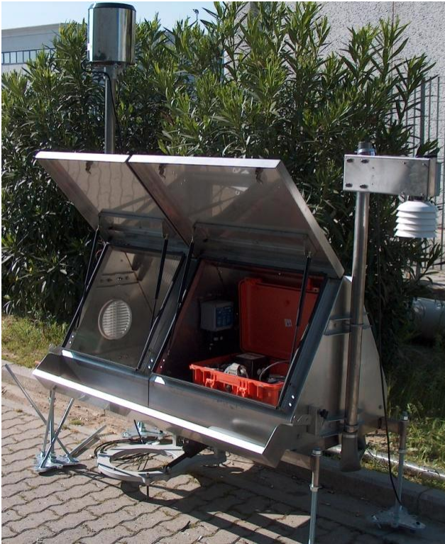
Fig. 1. The automatic measurement equipment as installed at the MSW site.
