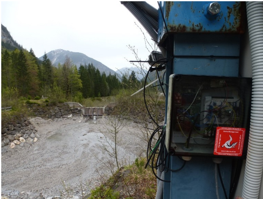
Abb. 51: Dristenau – Monitoring Station 1 Datenbox
