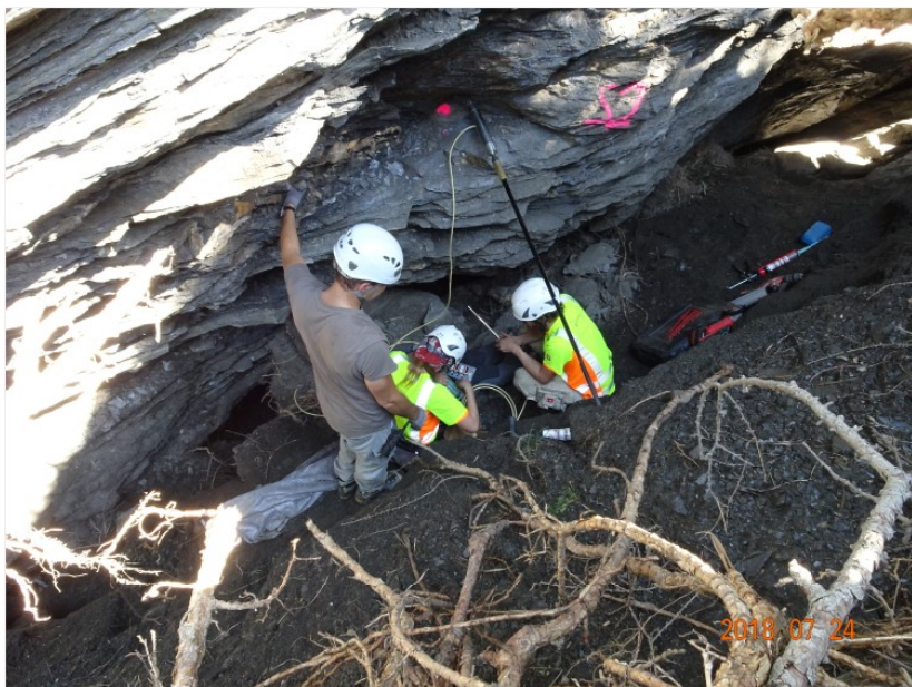
Abb. 32: Vals – Installation Crackmeter
