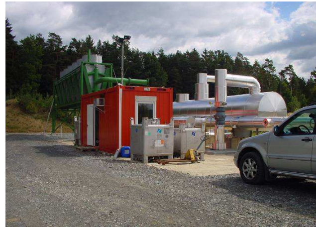
Blumau - ORC electricity facility
