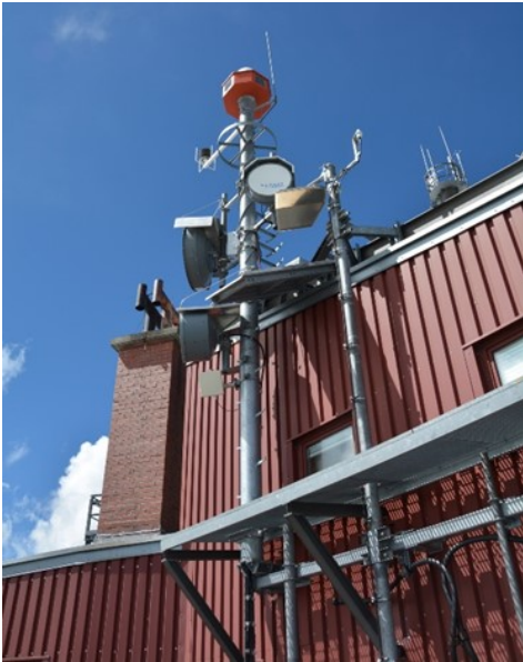
Standort: Empfangsantenne Location: Receiving antenna Quelle/Source: E. Ludewig@GEOSPHERE-AUSTRIA-SBO
