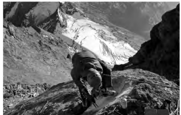
FIGURE 8: Drilling of a shallow borehole for iButton® temperature measurement at the Kitzsteinhorn south face (Photograph by Ingo Hartmeyer).
