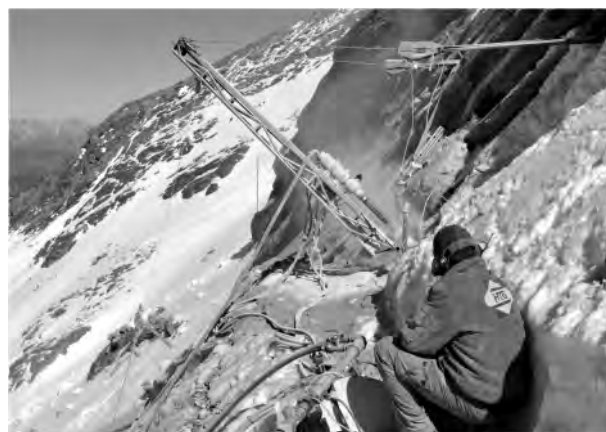
FIGURE 5: Air flush rotary drilling at the Kitzsteinhorn west face in September 2010 (borehole depth 30 m) (Photograph by Ingo Hartmeyer).
