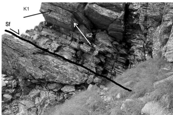
FIGURE 7: Foliation (Sf, black line) in the upper part of the mass movement, dipping downslope, enabling in combination with two orthogonal vertical joint sets (K1 and K2) sliding on cleavage planes; Picture taken from behind the ridge.
