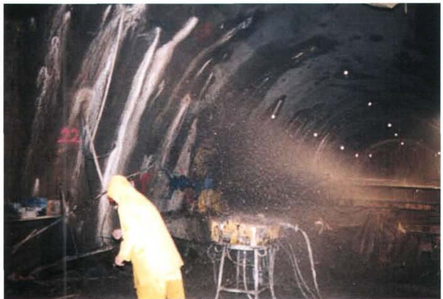
Fig. 9 A dramatic ingress of water (upper photograph) and sand- to gravel-sized dolomitic material (lower photograph), occurred after the drilling of anchor boreholes tapped a cohesionless water saturated fault zone at km 31.23, Brixlegg-East Reconnaissance Tunnel.
