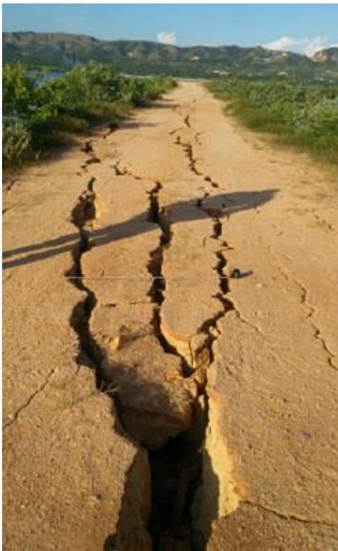
Figure 2. Cracking in natural soil road, VIII ESI-07 . Salina Cruz, Oaxaca.
