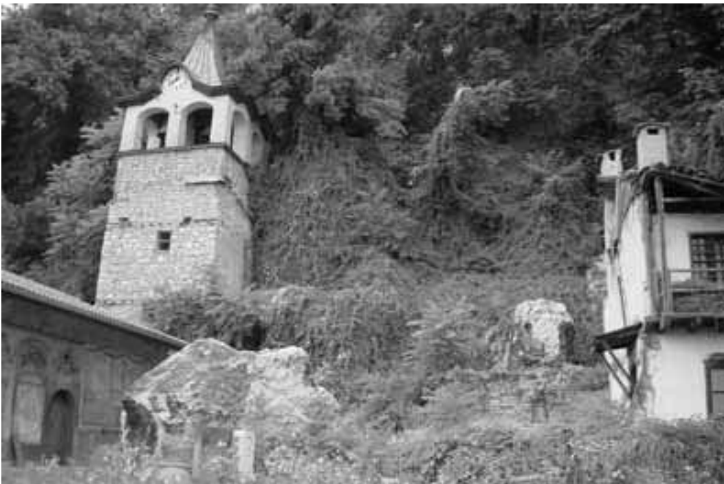
Figure 15 - View of the Monastery after the rock-fall
