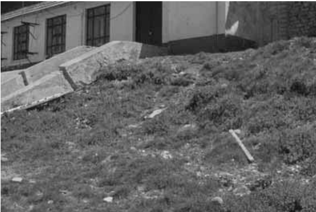
Figure 53 - The observatory entrance stairs cut by the Figure 54 scarplet.
