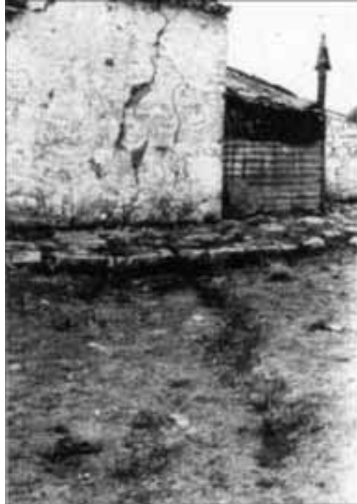
Figure 48 - Earthquake-induced ground fracture cutting a house
