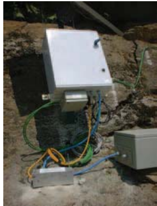
Figure 17 - Particular of micro-seismic data logger.
