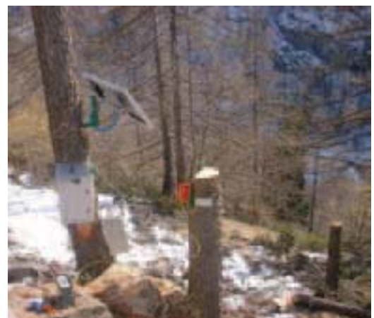
Figure 21 - Data logger of potenziometric extensometers' network.
