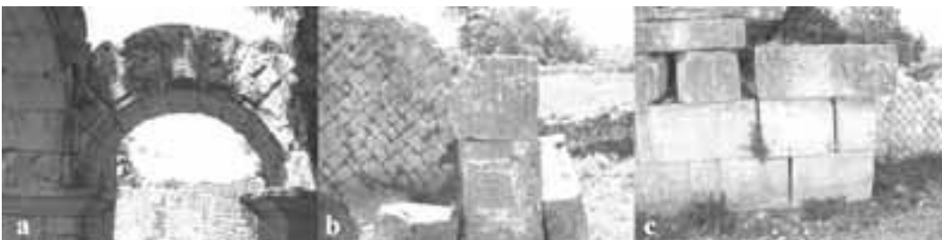
Figure 8 - Three examples of disconnected structures due to earthquakes: a) off-setting of lithons in an arc; b) block rotation in a pillar; c) increase of spacing between blocks in a wall.
